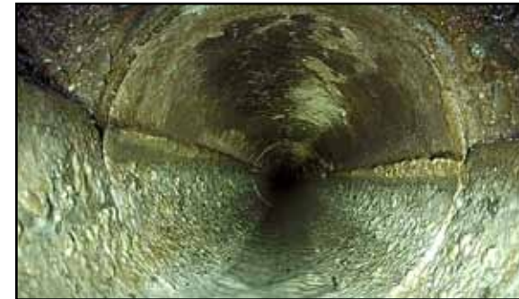
AN HD VIDEO NOZZLE IS RETRIEVED AT A RAPID SPEED UTILIZING HD VIDEO TO CAPTURE MAXIMUM PIPEWALL DETAIL.
