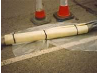
Liner folded for installation
