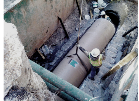
Above: The Hobas pipe was sliplined from the installation pit under the highway and railroad line.
