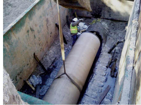
Above: Lightweight Hobas pipe can be lowered into the installation pit using only a canvas sling.
