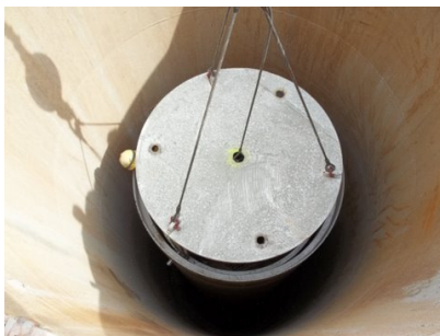
Left: A lightweight section of Hobas fiberglass liner is lowered into the shaft for installation.
