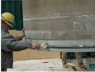
Left: Workmen apply lubricant to the gasket preparing it for quick push-together installation in the shaft.
